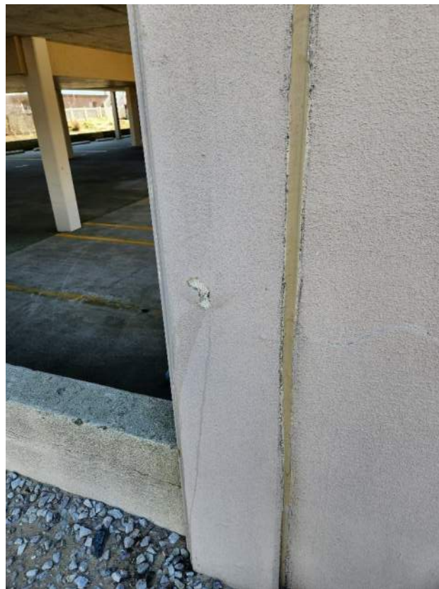
Photograph #22: North Façade Water Infiltration
