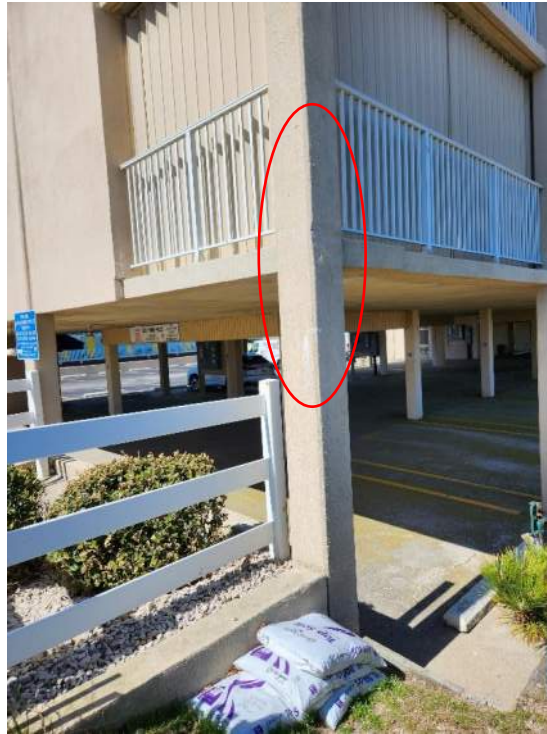
Photograph #19: Southeast Corner at Column Concrete Cracking
