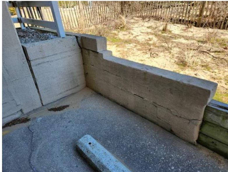
Photograph #8: Block Retaining Wall Cracking
