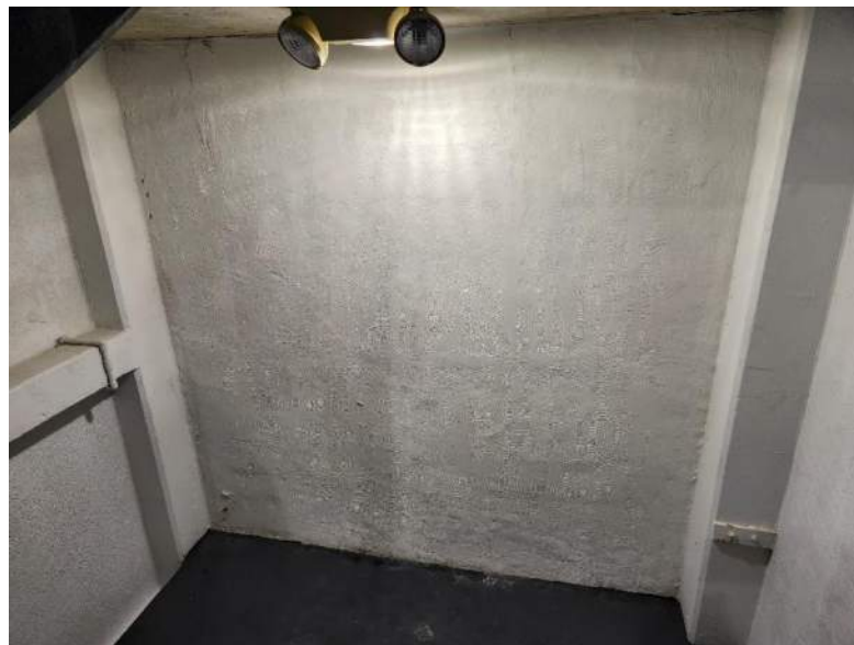
Photograph #16: Stair Tower Water Infiltration
