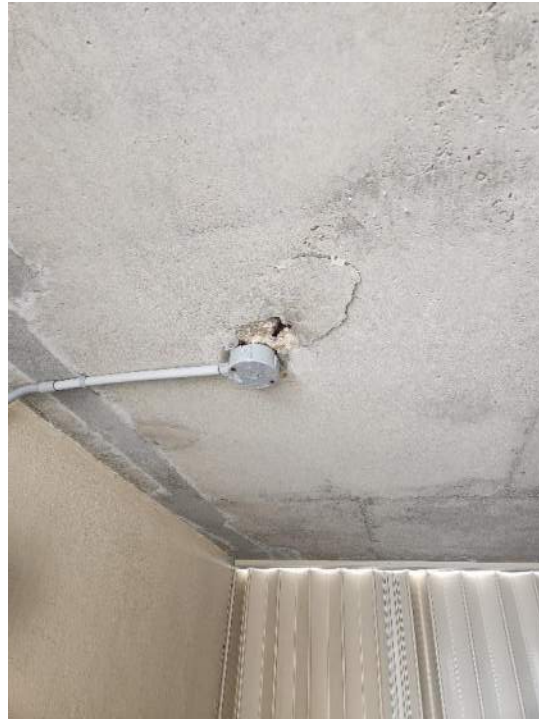
Photograph #15: Walkway Soffit Spall
