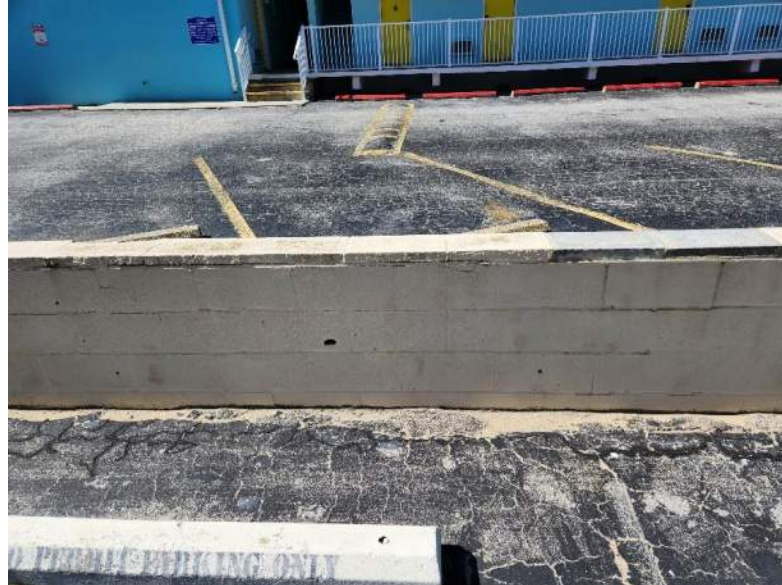
Photograph #7: Parking Area Landscaping Wall Cap Failure
