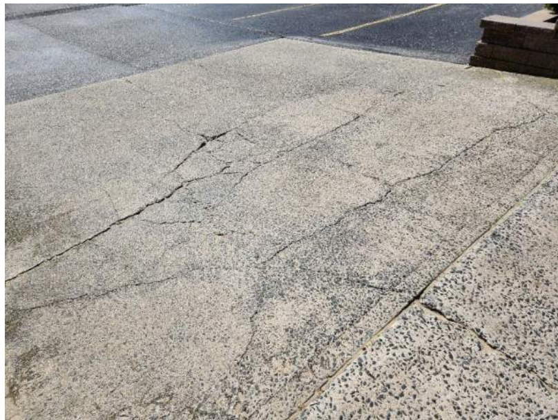
Photograph #4: North Entrance Slab Cracking
