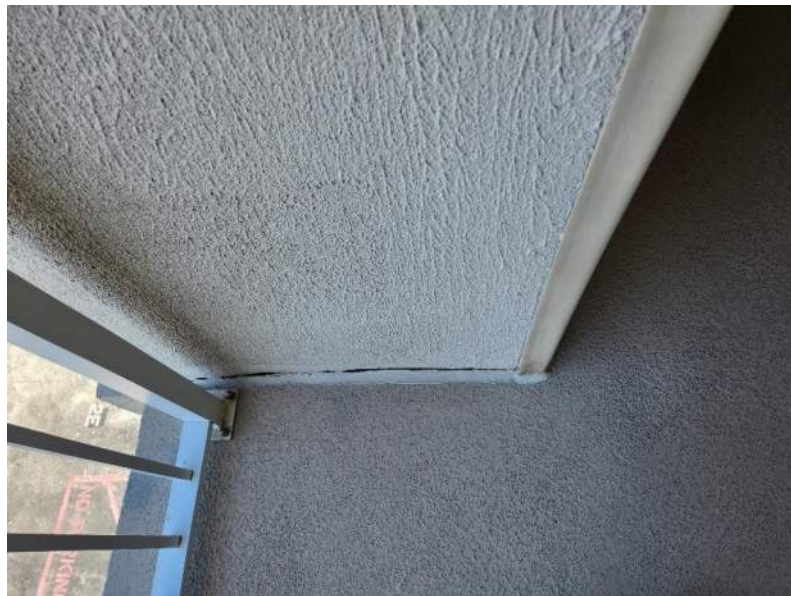
Photograph #14: Walkway Sealant Failure
