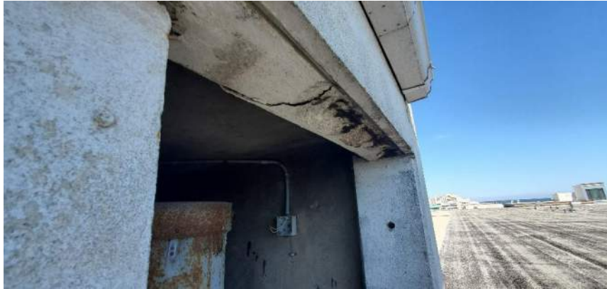
Photograph #25: Elevator Roof Lintel Failure
