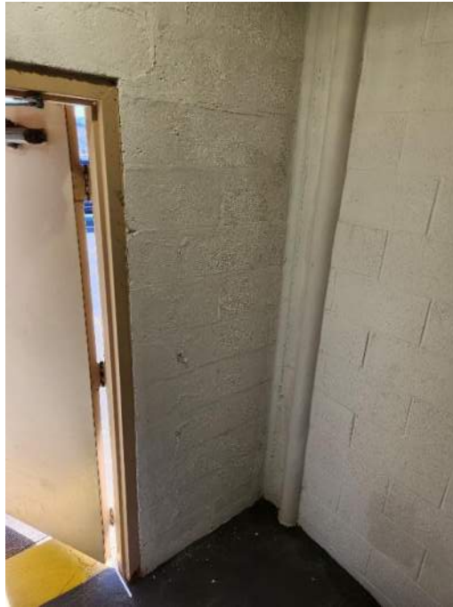
Photograph #17: Stair Tower Water Infiltration
