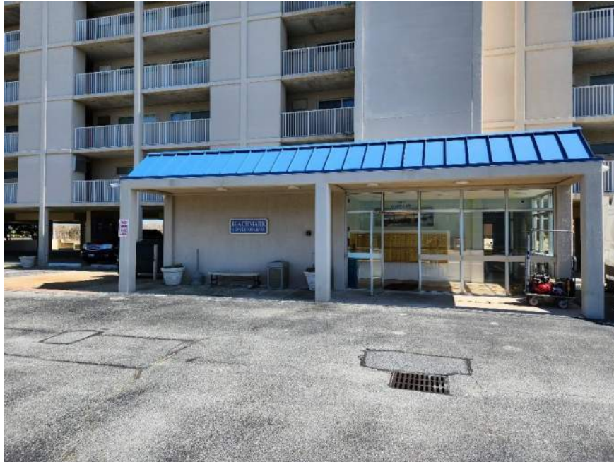
Photograph #9: Vestibule Aluminum Storefront
