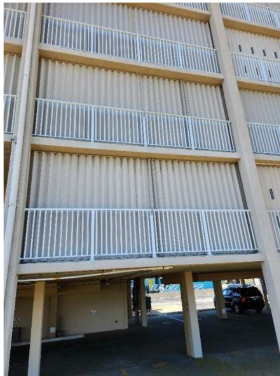
Photograph #20: East Façade Coating Failure
