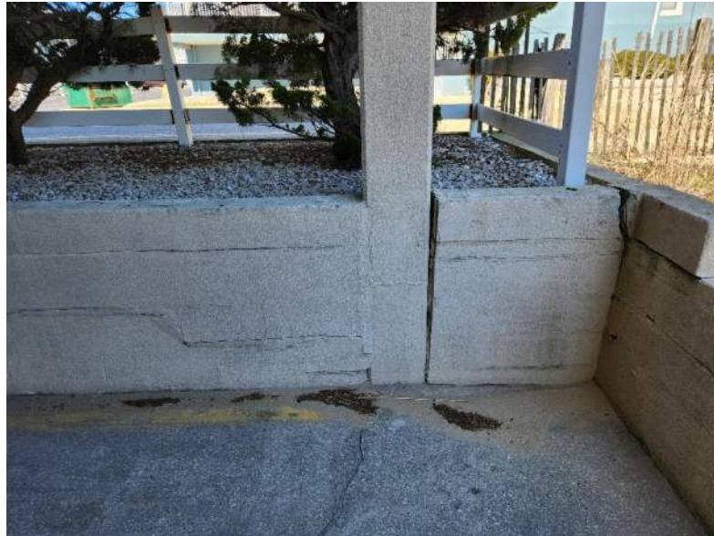
Photograph #21: Parking Area Retaining Wall Cracking
